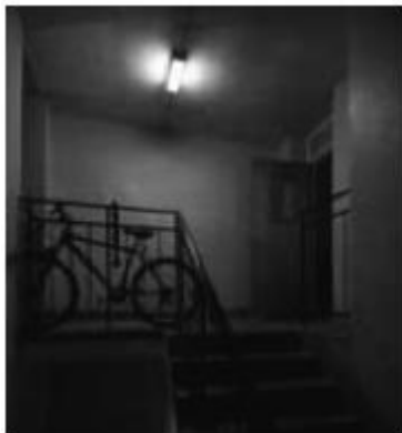
photo of stairwell with fluorescent fitting
