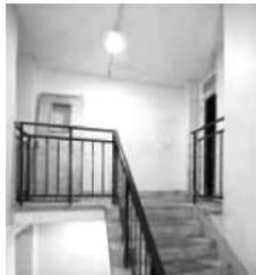
photo of stairwell with LED fitting
